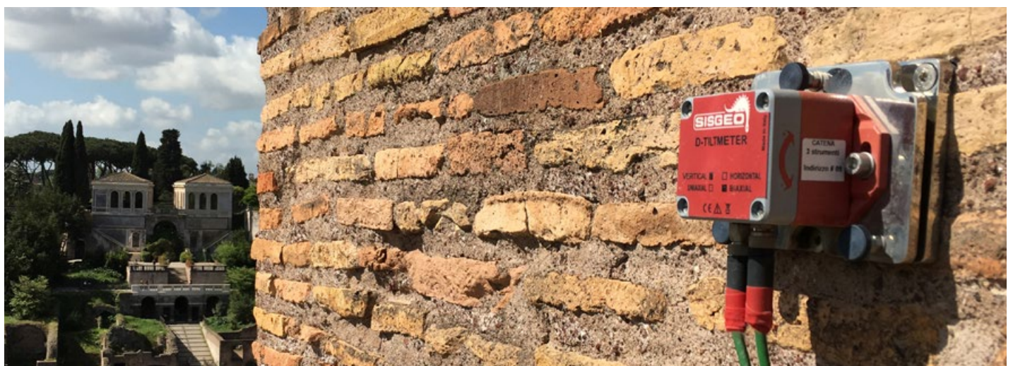
Tiltmeter installed on "Basilica di Massenzio", Rome - Italy
